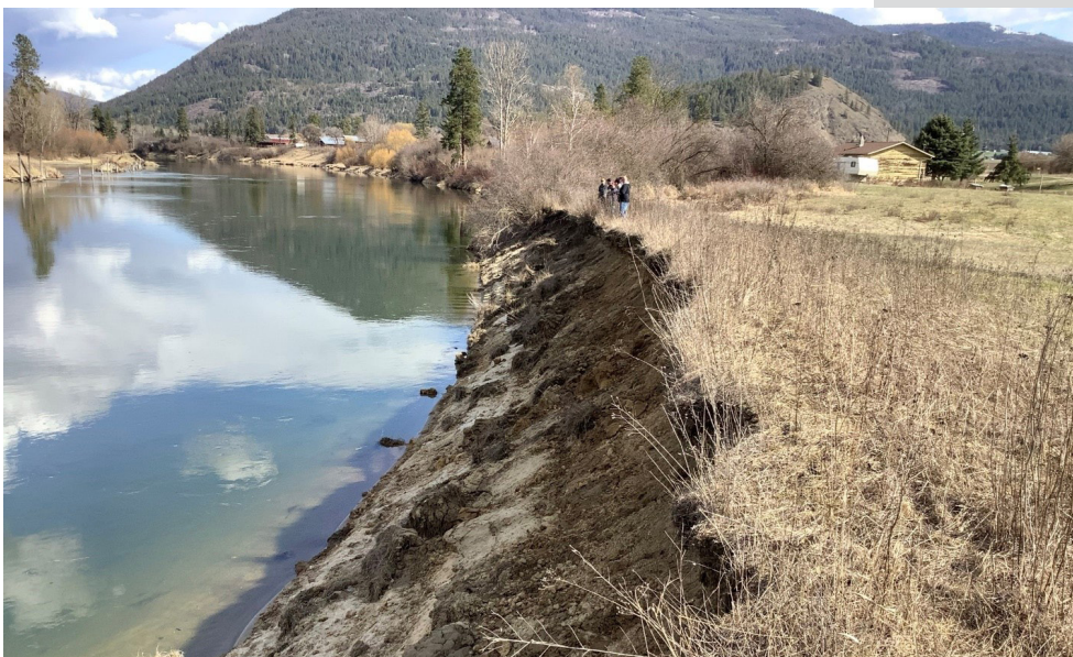
Bank erosion restoration site candidate assessed during a project team site visit conducted on March 26, 2024.
